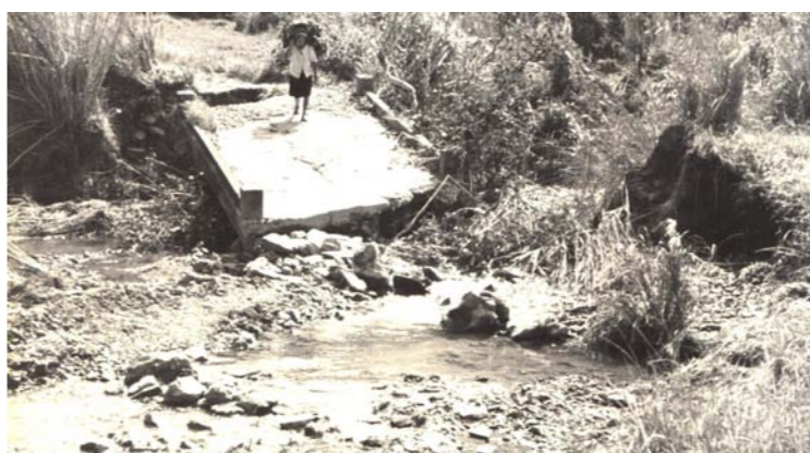
饒波橋梁決壊流失
